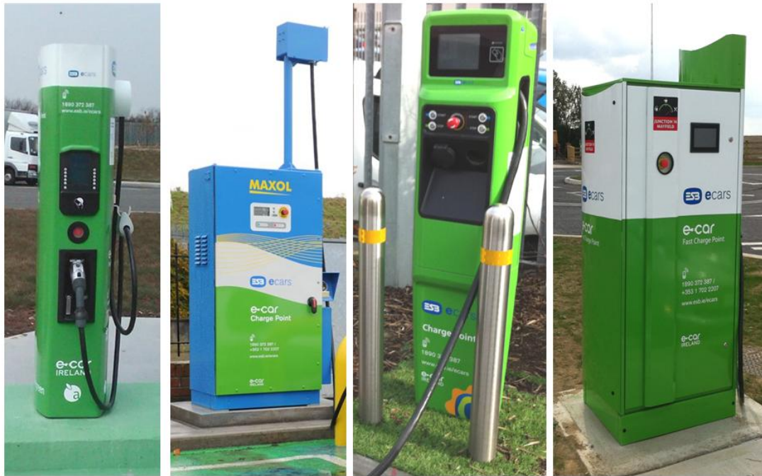
Figure Samples of Installed Fast Charge Points
